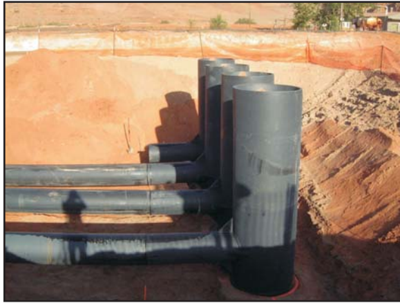
The four wet wells, prior to backfilling, that are associated with the river water storage pond.
